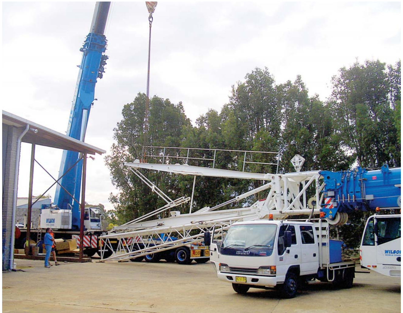
The operation, erection and dismantling of cranes require a fall protection plan as with any situation involving working at heights.
